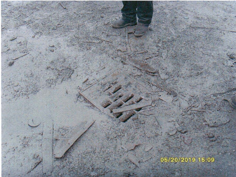
Photo 12 (SI850994): Drain located near the E-Z Crusher that Mr. McMilian said routes to the oil-water separator.
