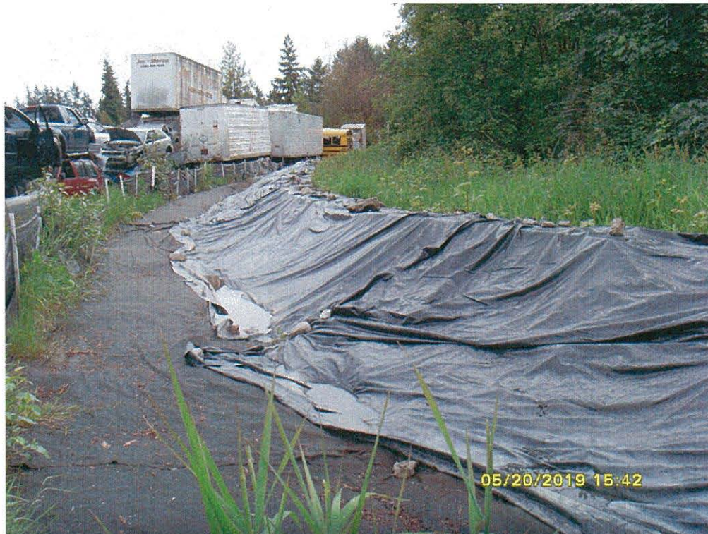
Photo 16 (SI851007): Southern view of the trench and berm near the northwestern corner of the facility yard.
