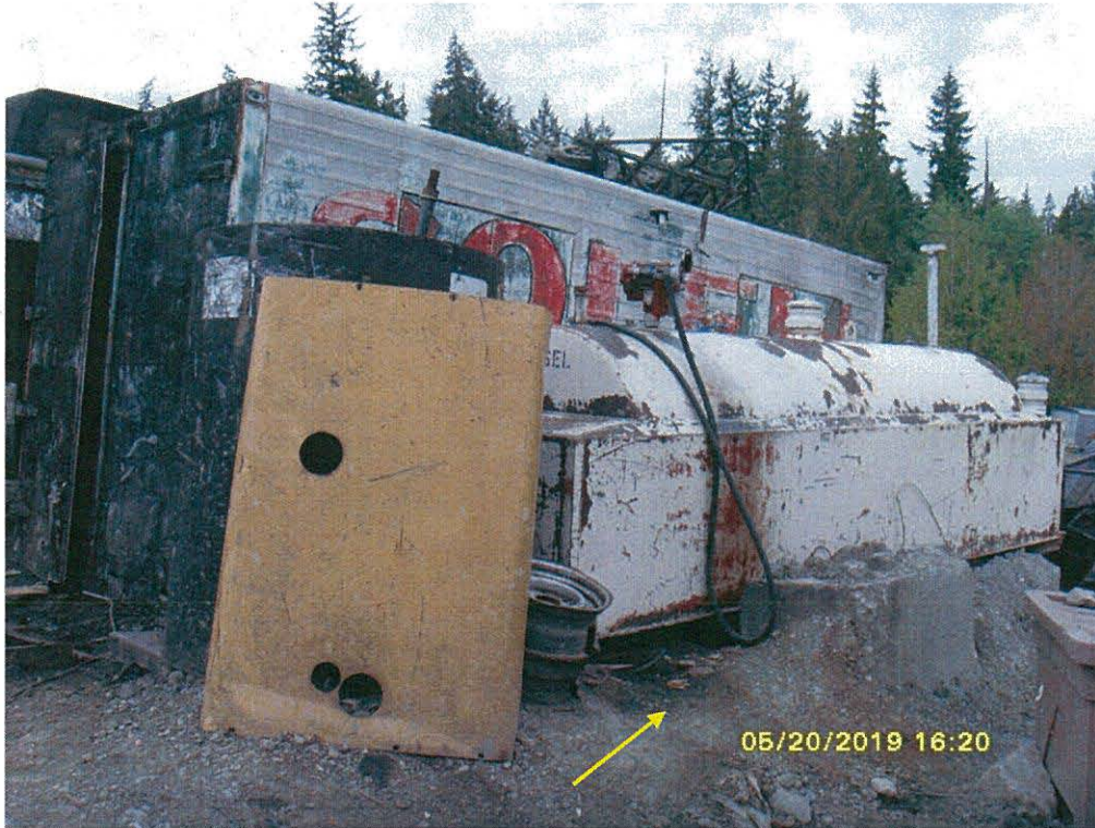
Photo 9 (SI851029): A 1,000-gallon diesel fuel tank located southwest of the main building and close to the E-Z crusher with staining on the side of the tank and beneath the tank (yellow arrow). According to facility representatives, this tank is double-walled.
