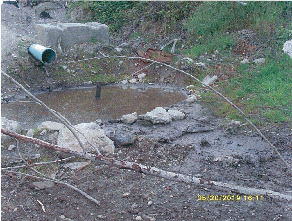
Photo 25 (SI851025): A pipe with fluid flowing from it, standing water, and staining located near the south end of the facility. According to facility representatives, the pipe routes drainage from the recently installed oil-water separator and catch basin located near the crushing pad.
