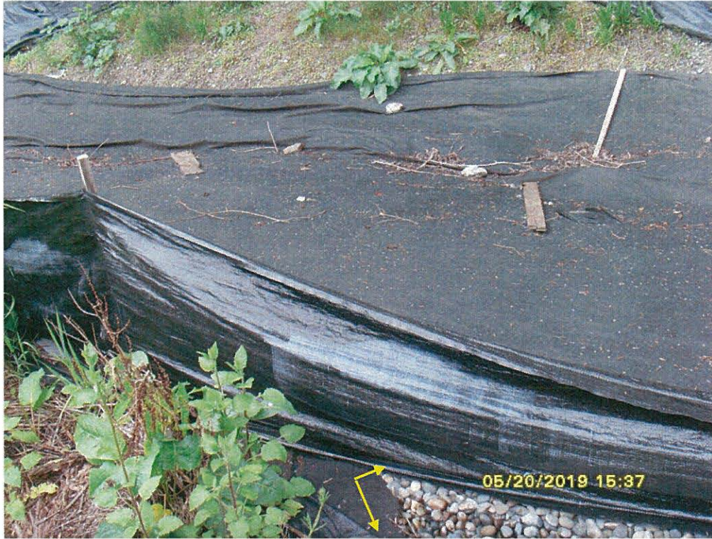
Photo 15 (SI851005): Northern view of the trench at the north end of the facility yard. Note that the sediment fencing is not installed correctly to make it effective at reducing sediment (yellow arrows).
