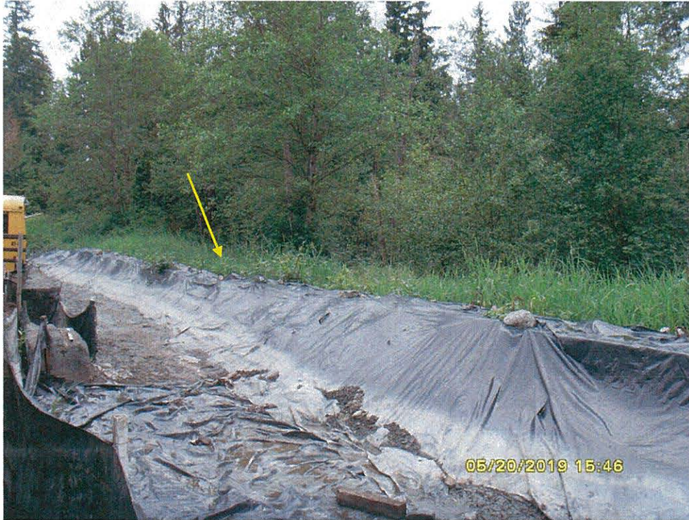
Photo 17 (SI851010): Southwestern view of the trench and berm at the west side of the facility yard. Mr. McMilian said that the facility has collected stormwater samples of a discharge from this approximate area (shown by a yellow arrow) in the past, when stormwater flows have overtopped the berm.
